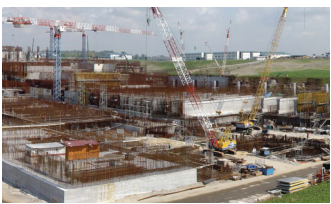
PUB Changi Water Reclamation Plant
