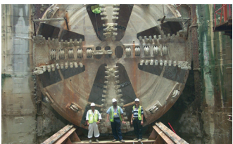
PUB Deep Tunnel Sewerage System (DTSS)
