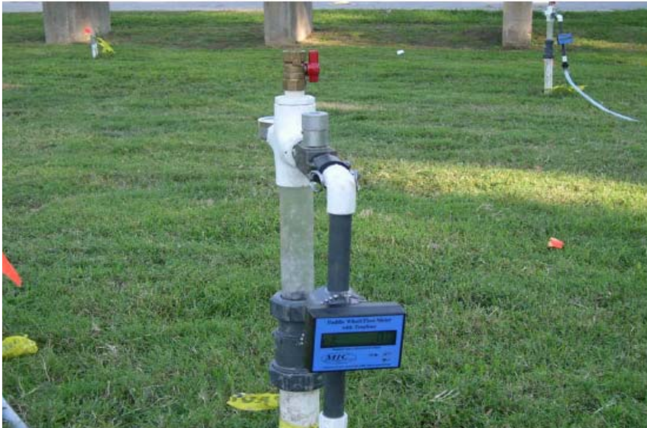
Newman Zone Injection Well with Digital Flowmeter
