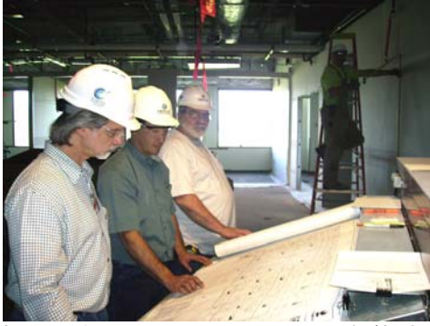
Construction Manager Joe Jurosky/CVO, Emerick Project Manager Mike Williams, and Emerick Project Superintendant Joe Aljets (left to right) review construction plans.
